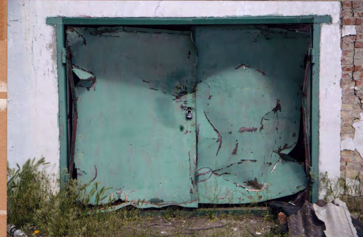
Curved gate to the garage after the blast. Borodianton
