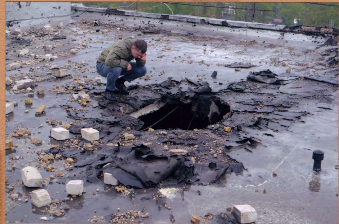
The Hole in the roof of a residential building after shelling IRPIN
